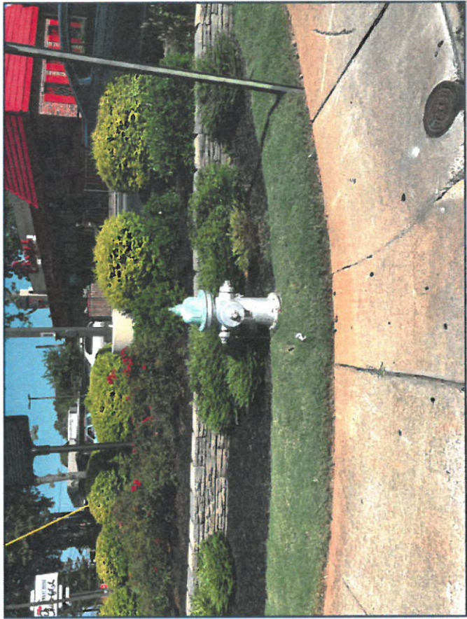
8 - Hydrant @ N Central Ave & Sherman Road
