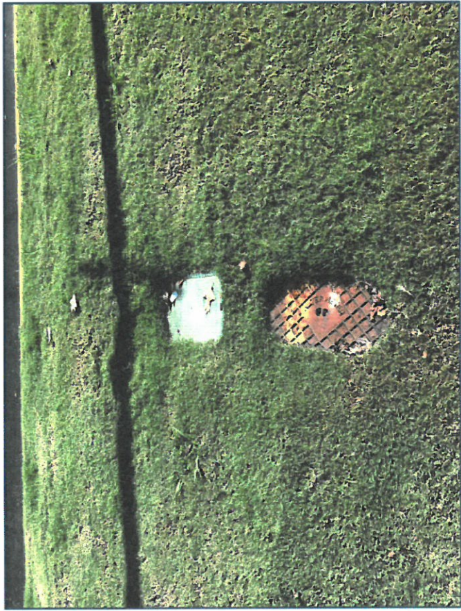
7 - Irrigation Meter Along N Central Ave
