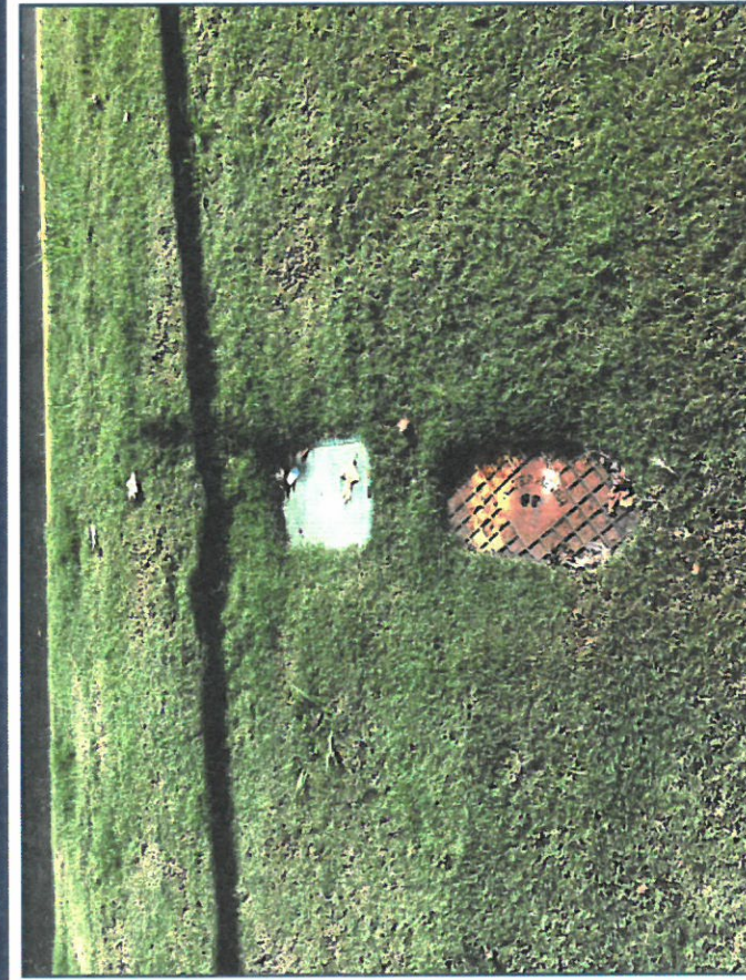
7 - Irrigation Meter Along N Central Ave
