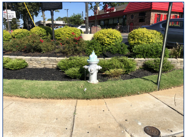
8 - Hydrant @ N Central Ave & Sherman Road
