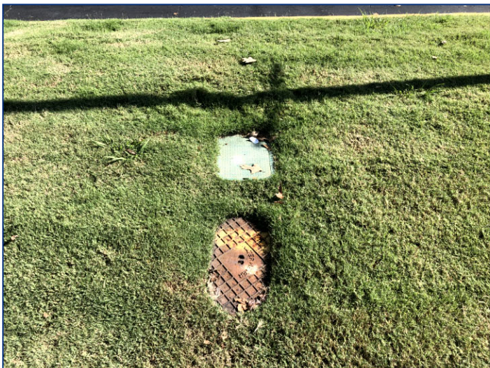
7 - Irrigation Meter Along N Central Ave
