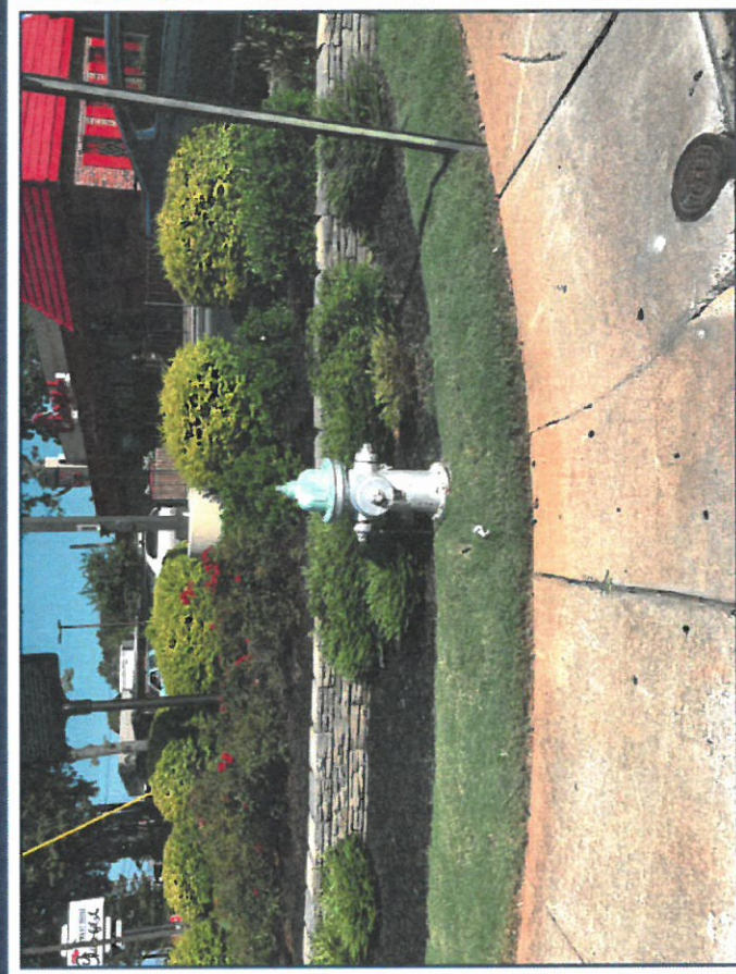
8 - Hydrant @ N Central Ave & Sherman Road
