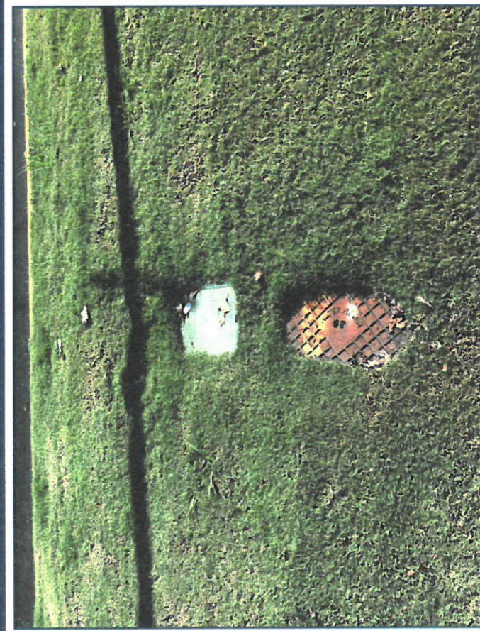
7 - Irrigation Meter Along N Central Ave
