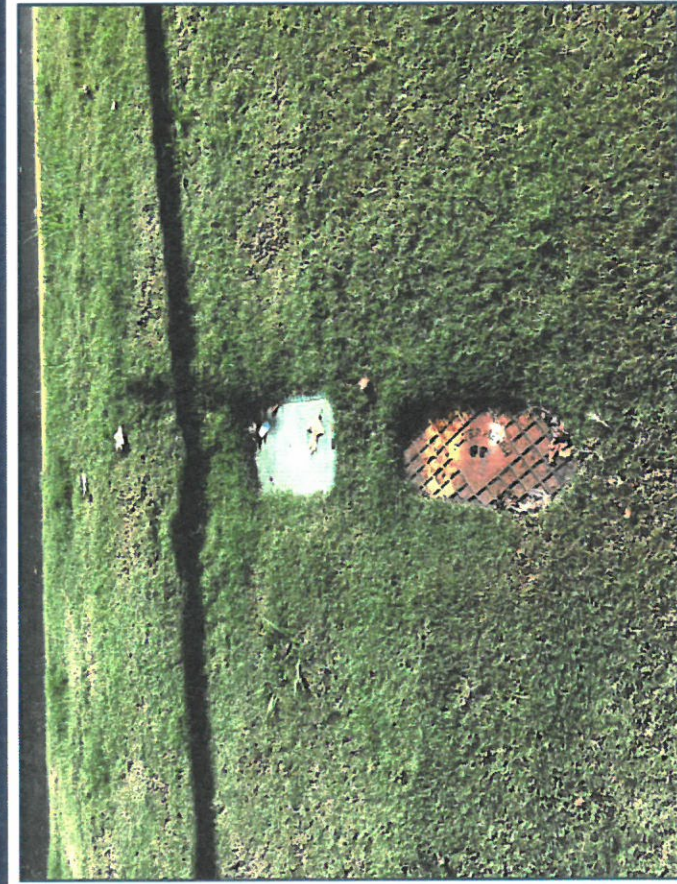
7 - Irrigation Meter Along N Central Ave
