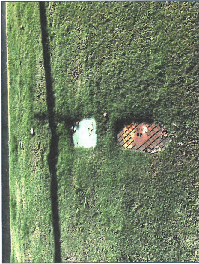
7 - Irrigation Meter Along N Central Ave
