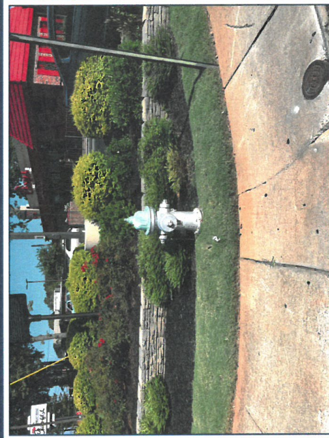
8 - Hydrant @ N Central Ave & Sherman Road
