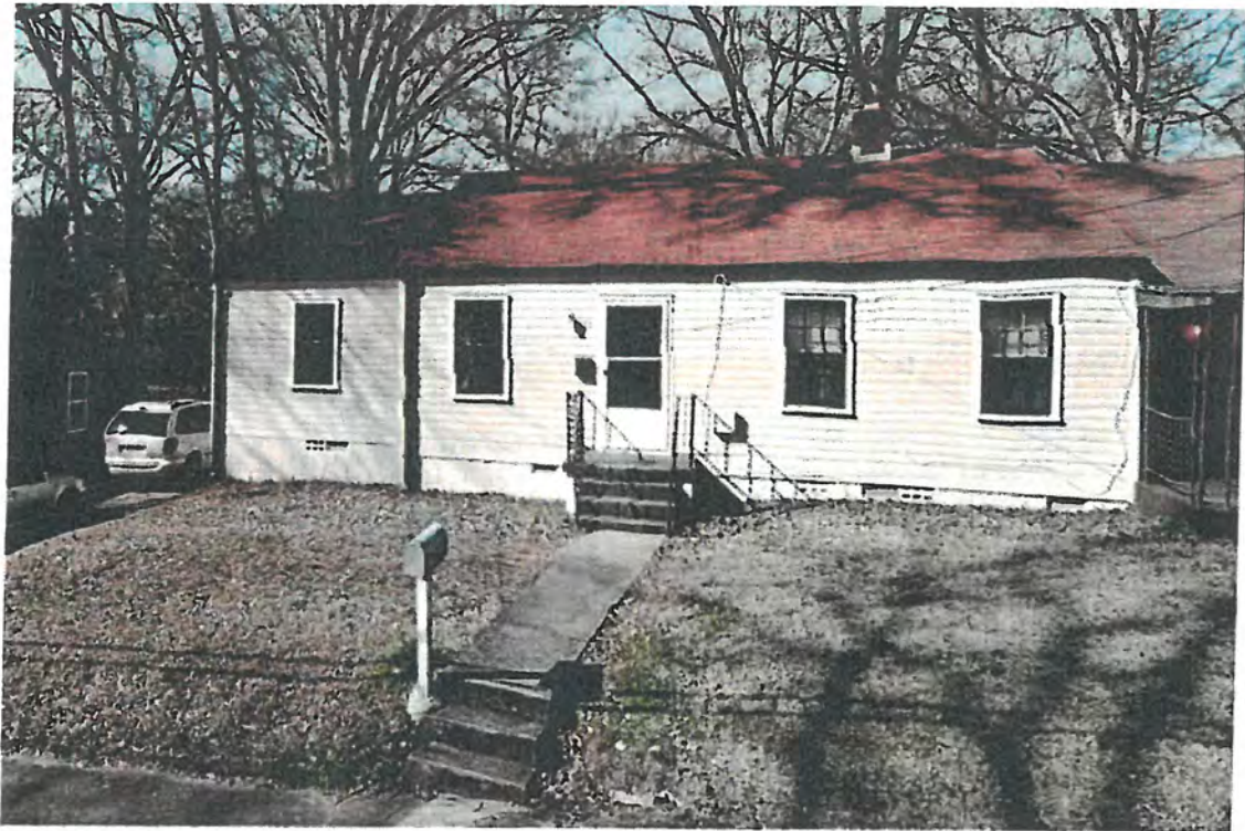
Before picture showing unlevel and cracked walkway
