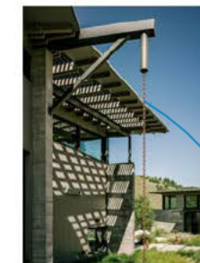
RAIN CHAIN + GUTTER
