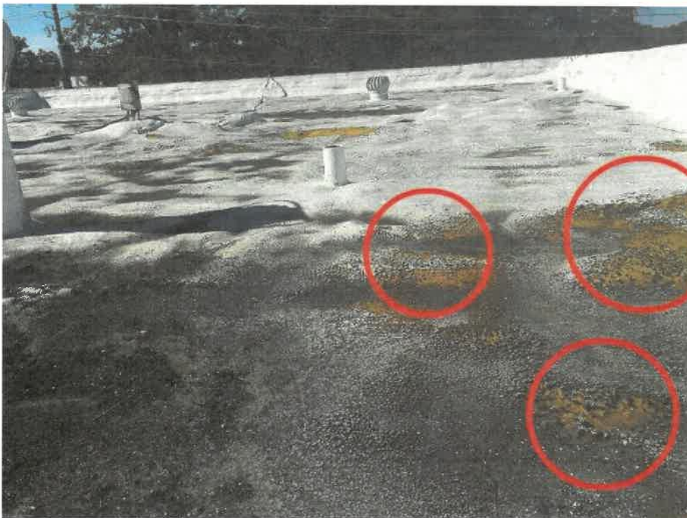
Red arrows show areas of exposed foam. This area will continue to breakdown due to PUF's weakness to UV light.
