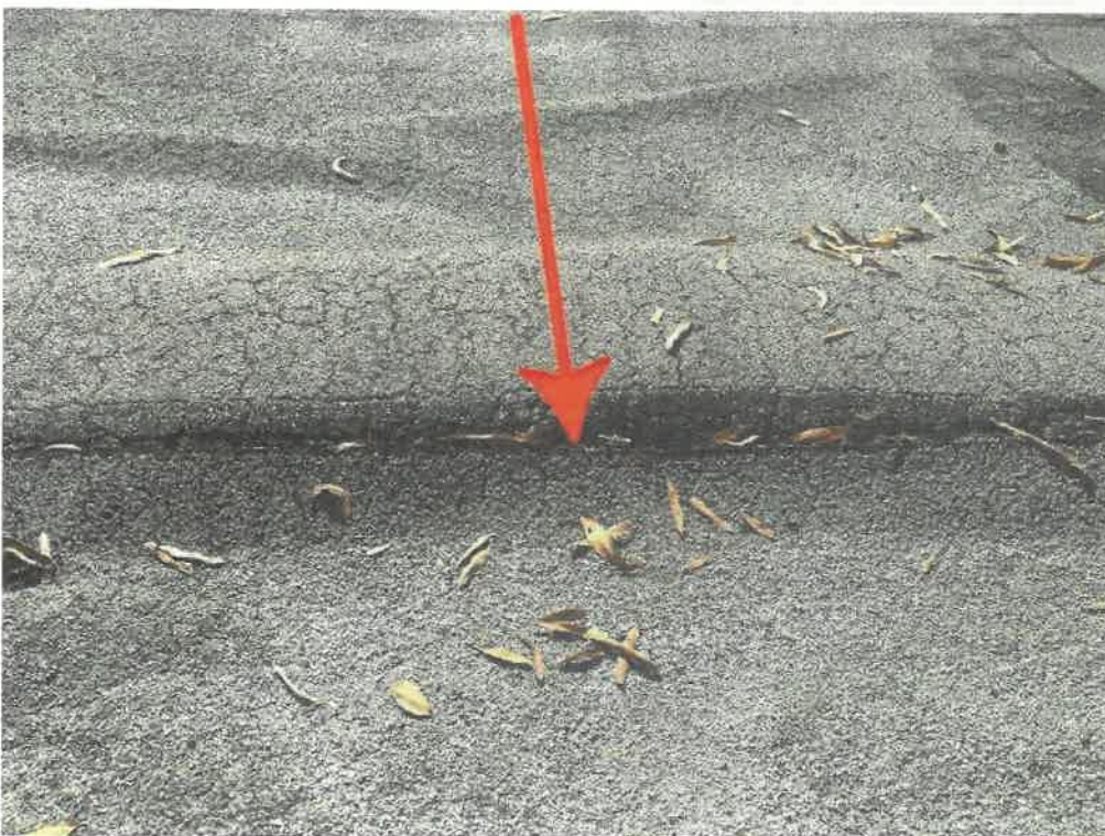
The red arrow shows a large blister directly on a seam. This blister will likely grow over time and continue to pull at the seam until it separates. At that time, it will allow a significant amount of water into the building.
