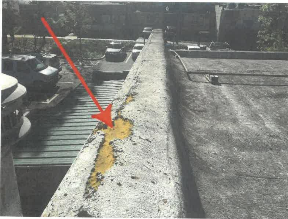
A large cavity in the PUF exposing the foam allowing water to penetrate the system.
