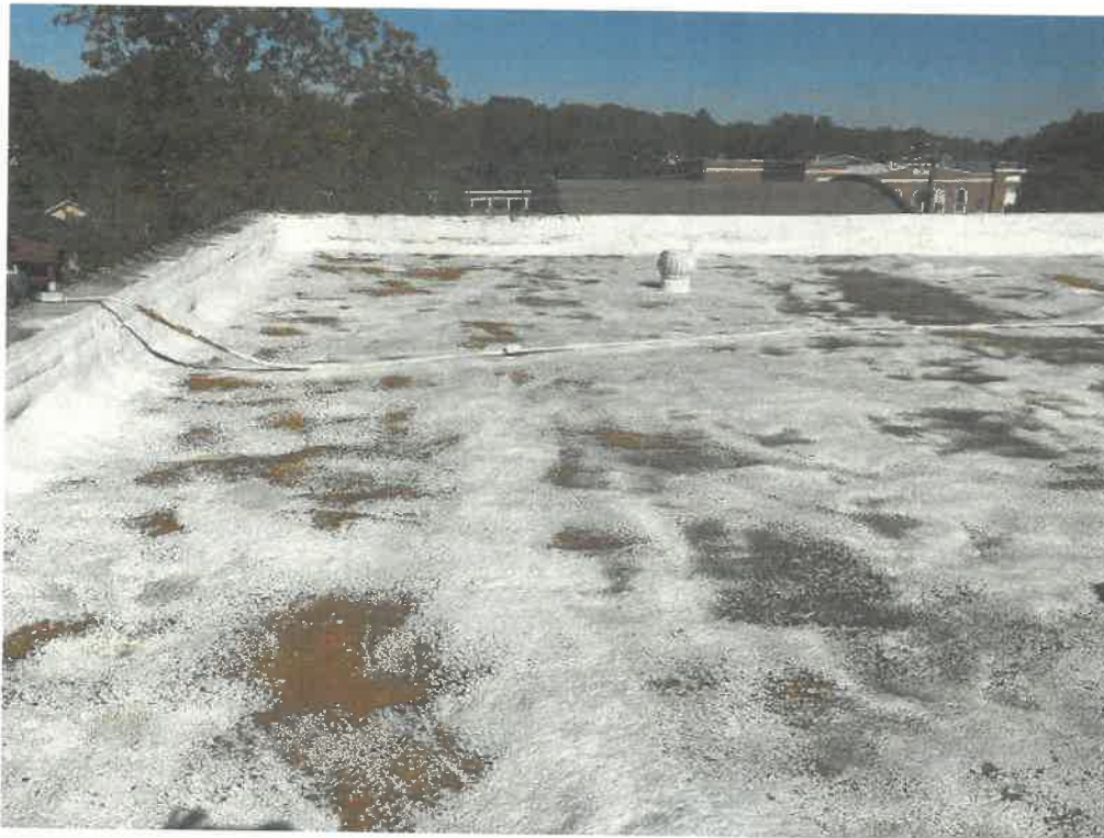
All areas that are not white, are areas that have failed and are no longer protecting the foam.
