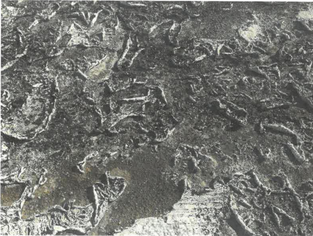
Close up of white coating peeling up.
